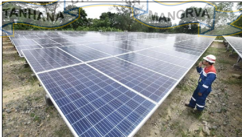
Gambar 4. PLTS Ground Mounted Badak Island, Kalimantan Timur
